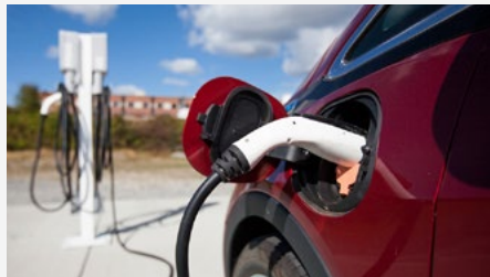
The EV charging station at Crane Aerospace & Electronics site in Lynnwood, WA.
